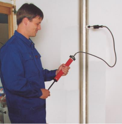
Fig. 4: Extracting the smoke gas
